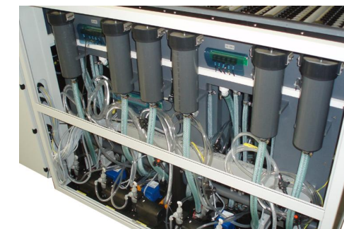
Specific filtration systems (incl software monitoring) for each individual tank according to the process requirements.
